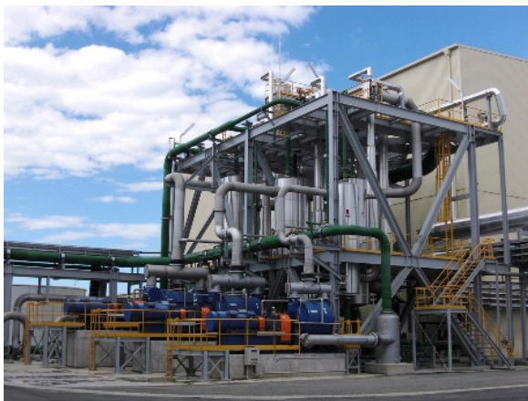
Figure 9: Photograph of Gas Extraction System
