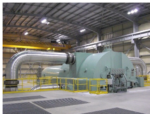
Figure 7: Photograph of Steam Turbine and Generator
