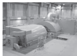
Reheating steam turbine
