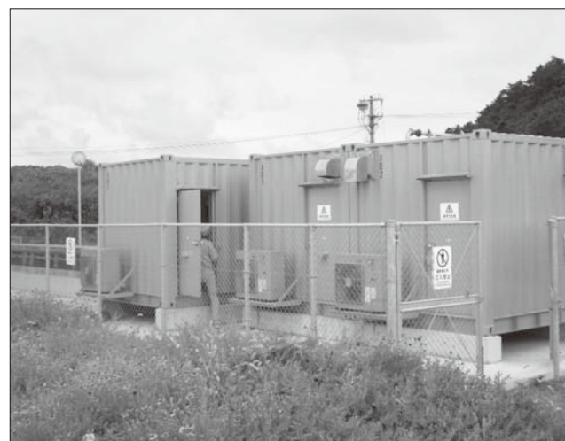
Fig.7 Appearance of storage containers
