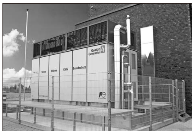
Fig.6 Fuel cell installed at Wismar
