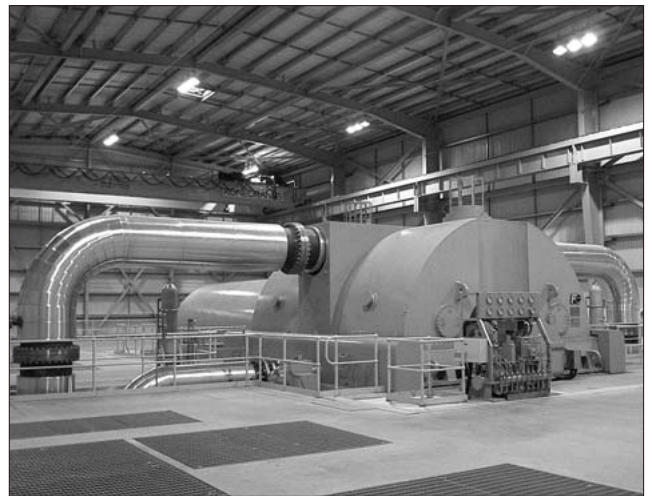
Fig.11 External appearance of the geothermal turbine for the NAP geothermal power station
