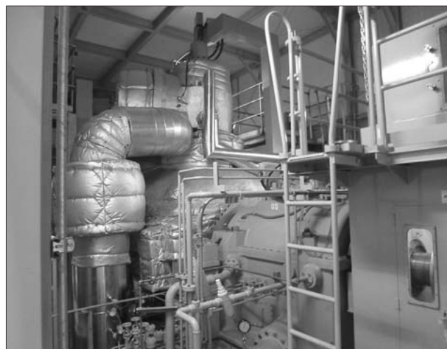
Fig.1 Steam turbine for Yoshinoura Thermal Power Station
