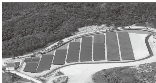
Fig.5 Overview of Abu mega-solar plant (Photograph supplied by the Okinawa Electric Power Company, Incorporated)
