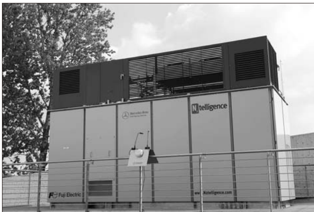
Fig.7 Fuel cell installed at Hamburg
