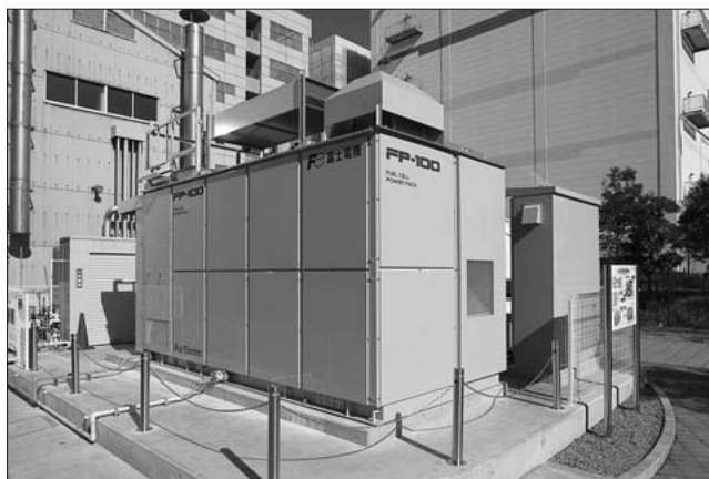
Fig.3 Fuel cells installed at Fuji Electric's Kawasaki Factory
