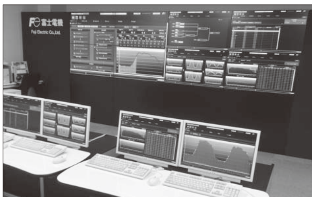
Fig.3 CEMS installed in the Community Setsuden-sho
