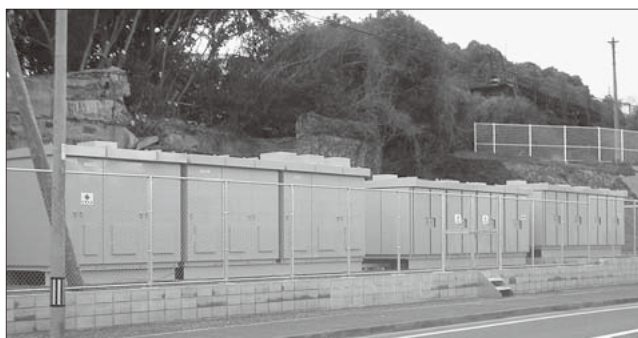
Fig.4 Storage system for 300 kW
