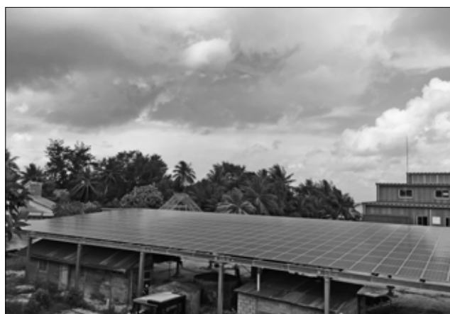
Fig. 3 Roof-type photovoltaic modules
