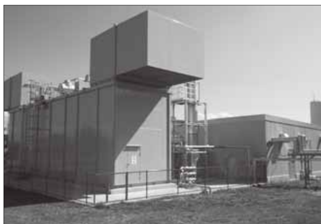
Fig. 11 External appearance of cogeneration system
