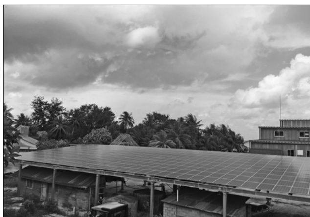
Fig. 3 Roof-type photovoltaic modules
