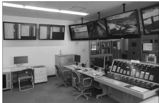
Fig.1 Dam discharge facility controlling equipment for Izarigawa Dam Control Center
