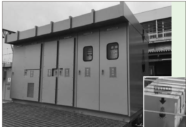
Fig.2 Direct current electric power converter
