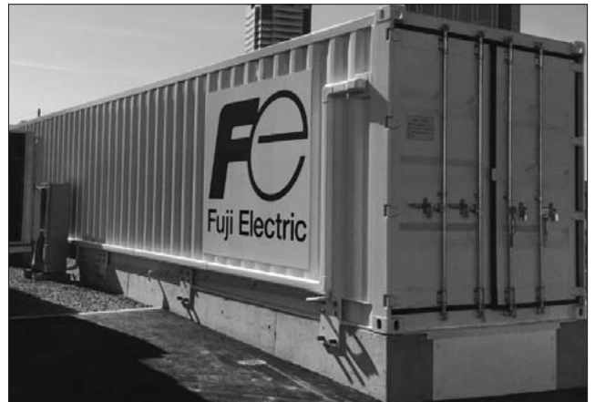
Fig.3 External appearance of large-scale lithium-ion battery facility
