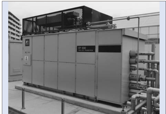
Fig.7 Fuel cell installed at Tokyo Factory
