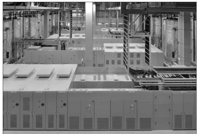
Fig.4 Installation arrangement of large-scale power conditioning systems
