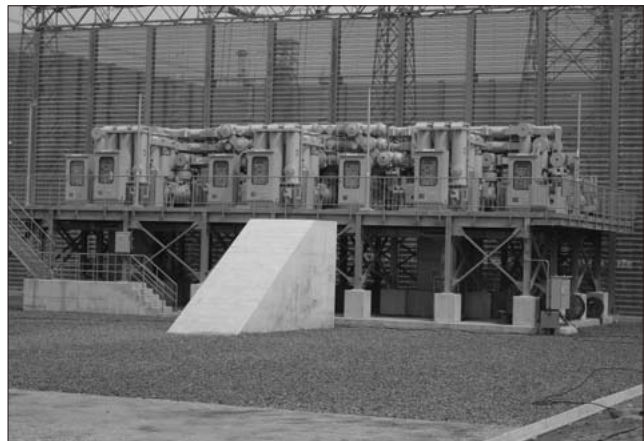
Fig.3 Shin-Sendai Thermal Power Station 300-kV GIS
