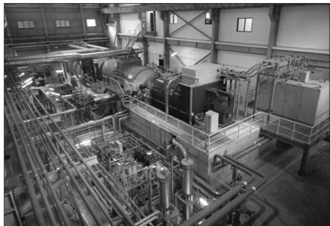
Fig.1 Steam turbine and generator
