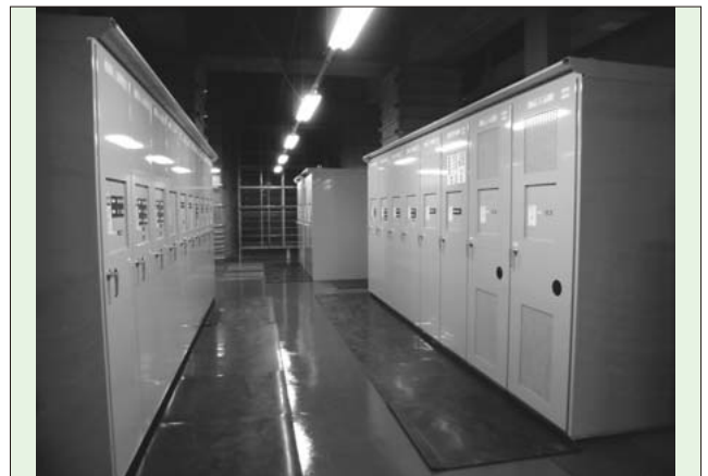
Fig.1 24-kV AC C-GIS and 1,500-V DC/7.2-kV AC enclosed switchgear
