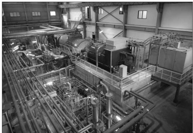
Fig.1 Steam turbine and generator
