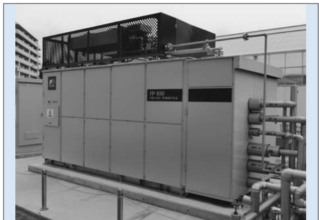
Fig.7 Fuel cell installed at Tokyo Factory
