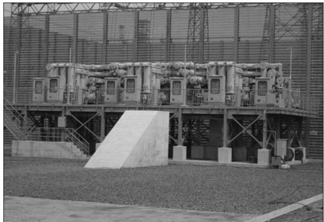
Fig.3 Shin-Sendai Thermal Power Station 300-kV GIS
