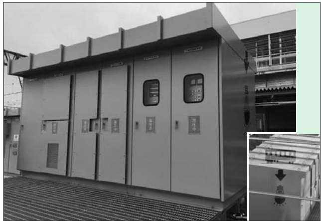
Fig.2 Direct current electric power converter
